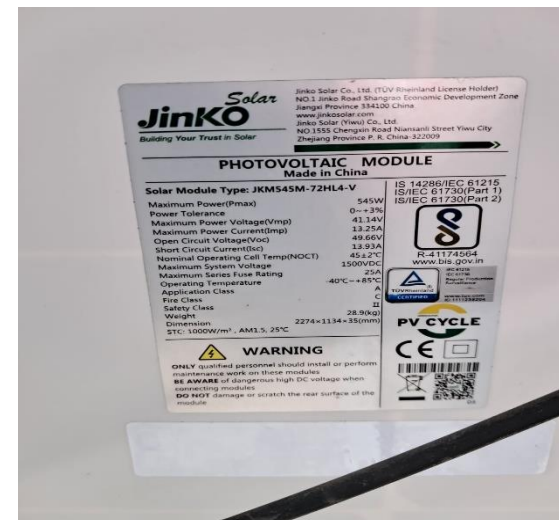
Figure 1 Actual photographs of installed Solar panels & name plate of power module
