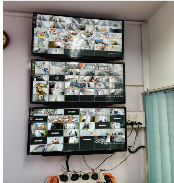
Figure 2 CCTV monitoring room
